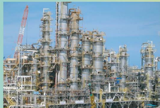
Pipings in processing plants are commonly inspected radiography methods
