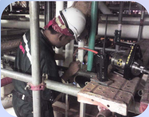
Radiography performed in confined areas above the ground in industrial plants if not planned properly may lead to overexposure.
