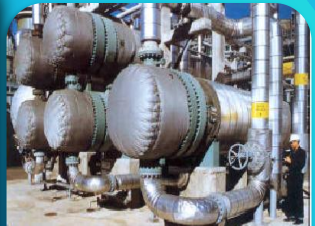
Complex structures such as shown in this picture have always been used as an excuse for high radiation exposure received by industrial radiographers.
